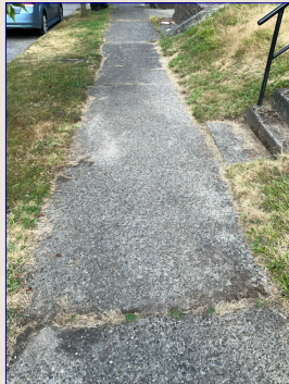
The Service Walk View
