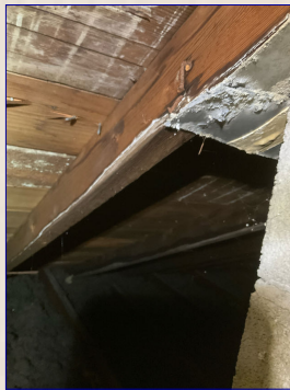
There is staining and evidence of prior moisture on the roof sheathing as viewed from the attic. No current moisture was detected during the inspection. Recommend monitoring and consulting a licensed roofer as needed.
