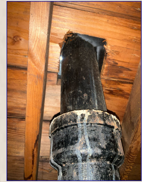
There is staining and evidence of moisture on the roof sheathing as viewed from the attic. Recommend a licensed roofer repair.
