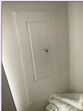
The main electrical service panel
