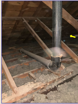
There is staining and evidence of moisture in the attic. Recommend a licensed roofer repair.
