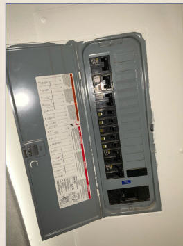
The main electrical service panel
