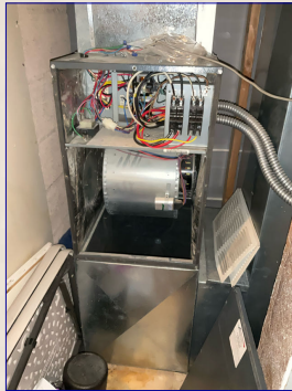
The furnace area
