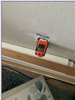
Electrical receptacle not operating
